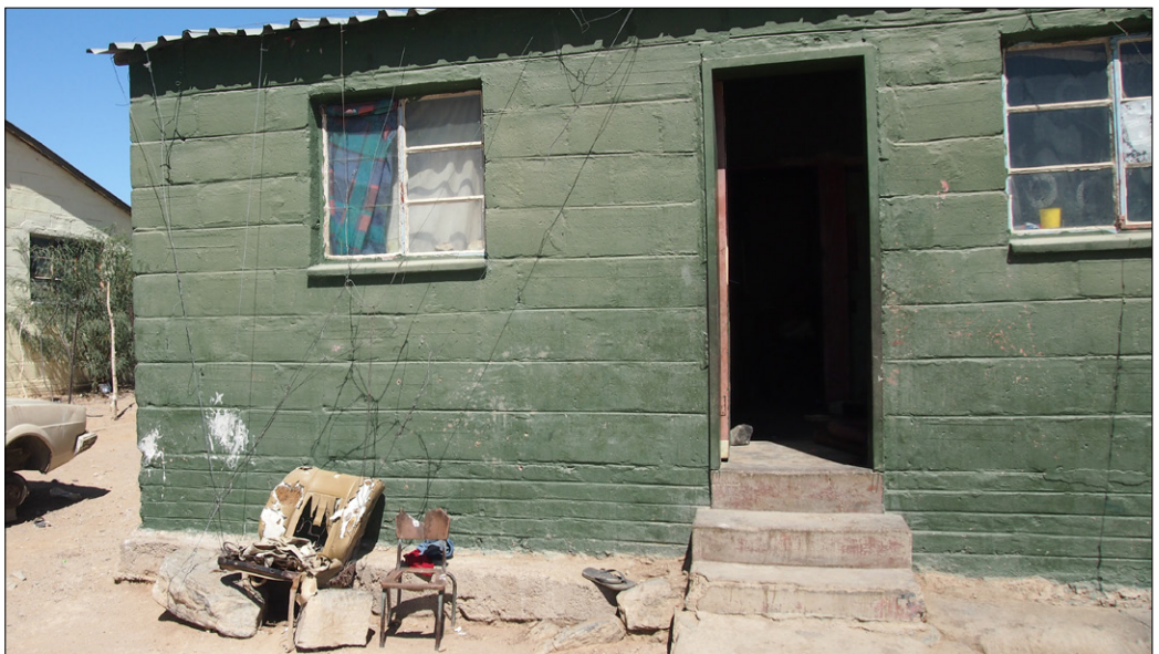
Mining left the community in Uis in poverty. Houses cracked and the roofs had to be re-inforced with wire. Source: Author
